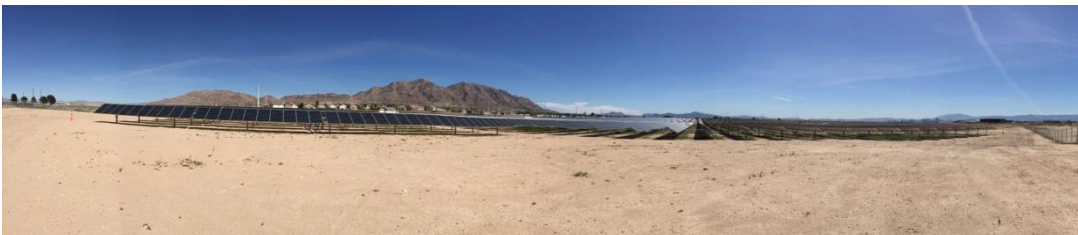
Large solar array at Nellis Air Force Base (Photo credit M. McCarthy)
