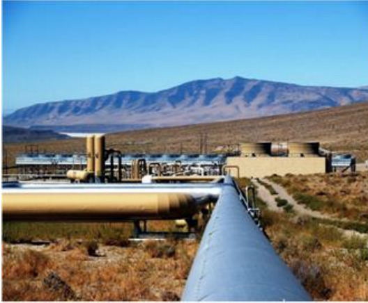
Figure 3. Nevada's Desert Peak 2 Geothermal Plant (Photo Credit Ormat Technologies)
